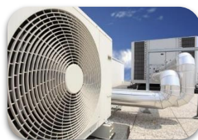
Heating and Cooling
